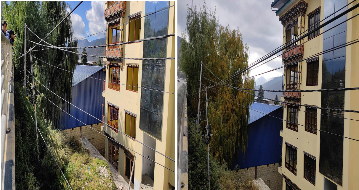
Figure 6: Improper cable layout near Babesa Zero/Junction, Before and After
