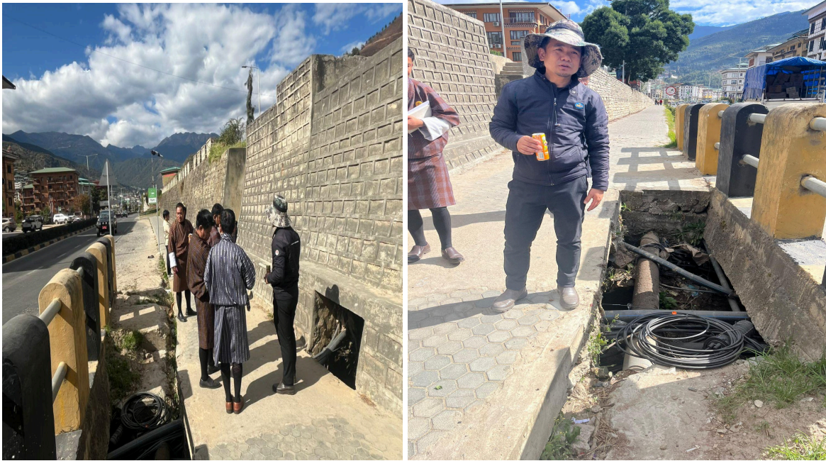
Figure 18: Common duct at near helipad
