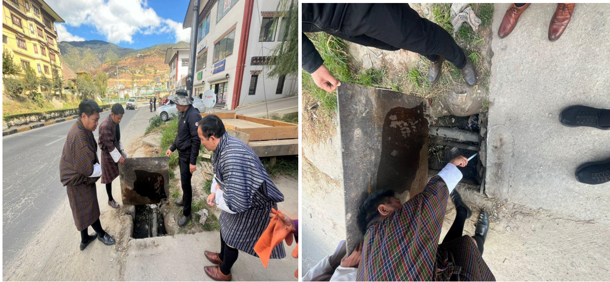
Figure 15: Common duct near O-plaza building
