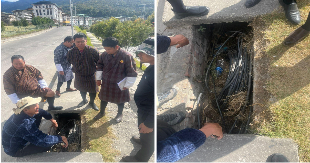
Figure 17: Common duct along Changjalu road
