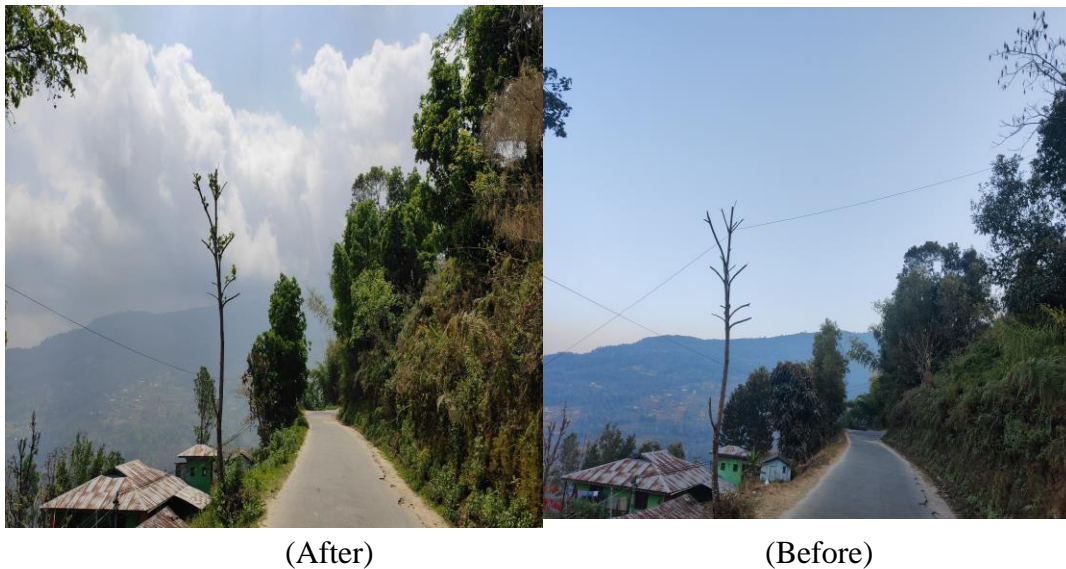
Figure 6: Road cross over in the peripheral area of Dagapela town by BTL and NL Cable is fixed.
