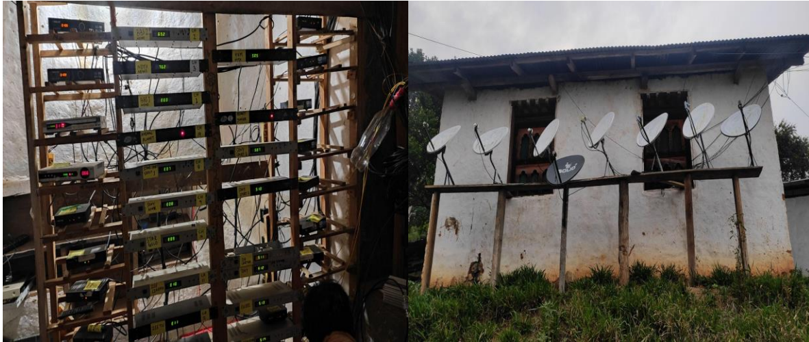
Figure 5: Norbu Cable Service control room.
