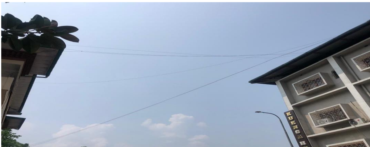
Figure 14: improper cable road crossover and improper cable layout of BTL and Tshela Cable Service below Zangdopelri road crossover
