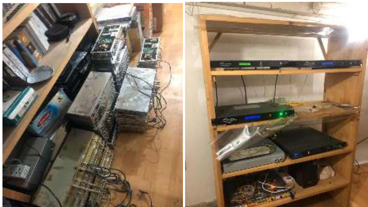
Figure 1. Control Room of Leki Cable Service, Haa
