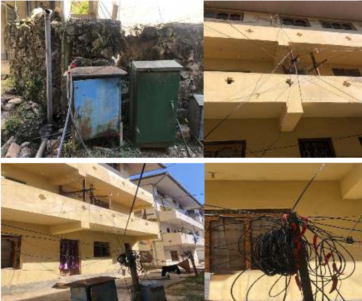
Figure 9. Improper Cable Layout
